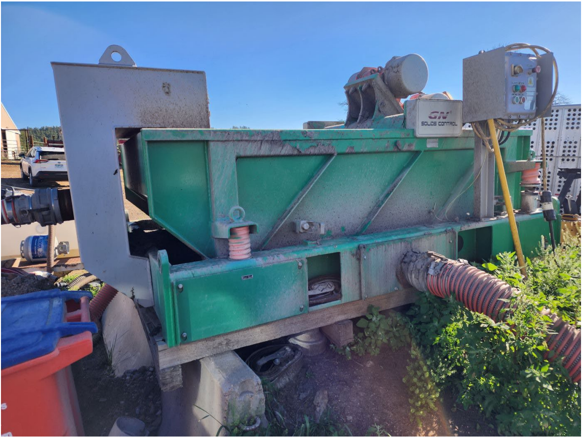
Photo 1: Shaker screen used to remove debris from septage.
