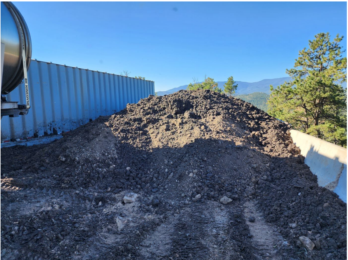
Photo 6: Solids stored behind the dewatering unit.
