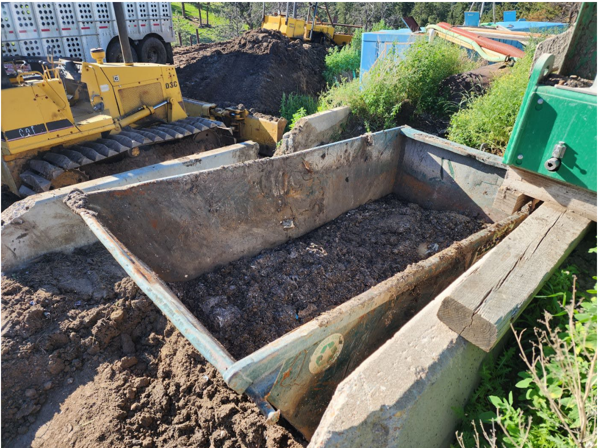
Photo 2: Bin for collection of debris screened from incoming septage.
